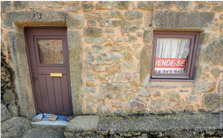
Many regions in Europe suffer from land abandonment and young generations moving to cities, with significant socio-economic impacts for rural areas. Abandoned house in Castelo Rodrigo, Portugal.
