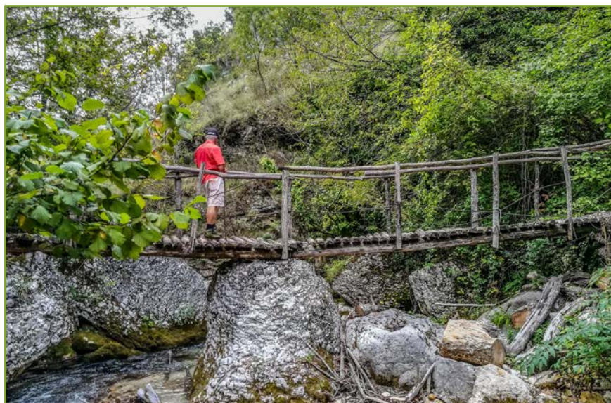
Fig. VIII-28: There is permanent infrastructure necessary for tourism activities in the Restoration zone.
